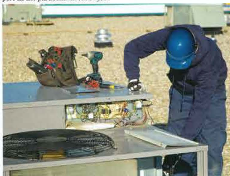
Larger restaurant facilities with high demand on HVAC, for example, will benefit from a BMS.
